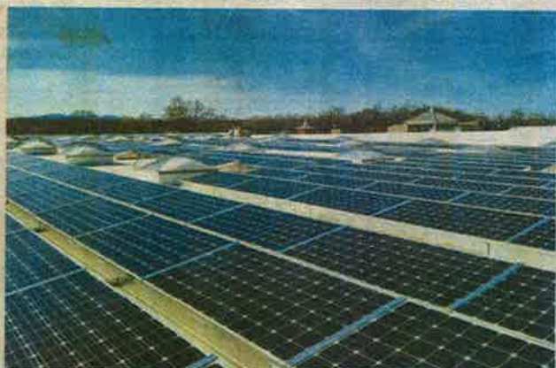
Solar panels have been installed on the roof of the Rhinebeck Stop & Shop. COURTESY PHOTO
