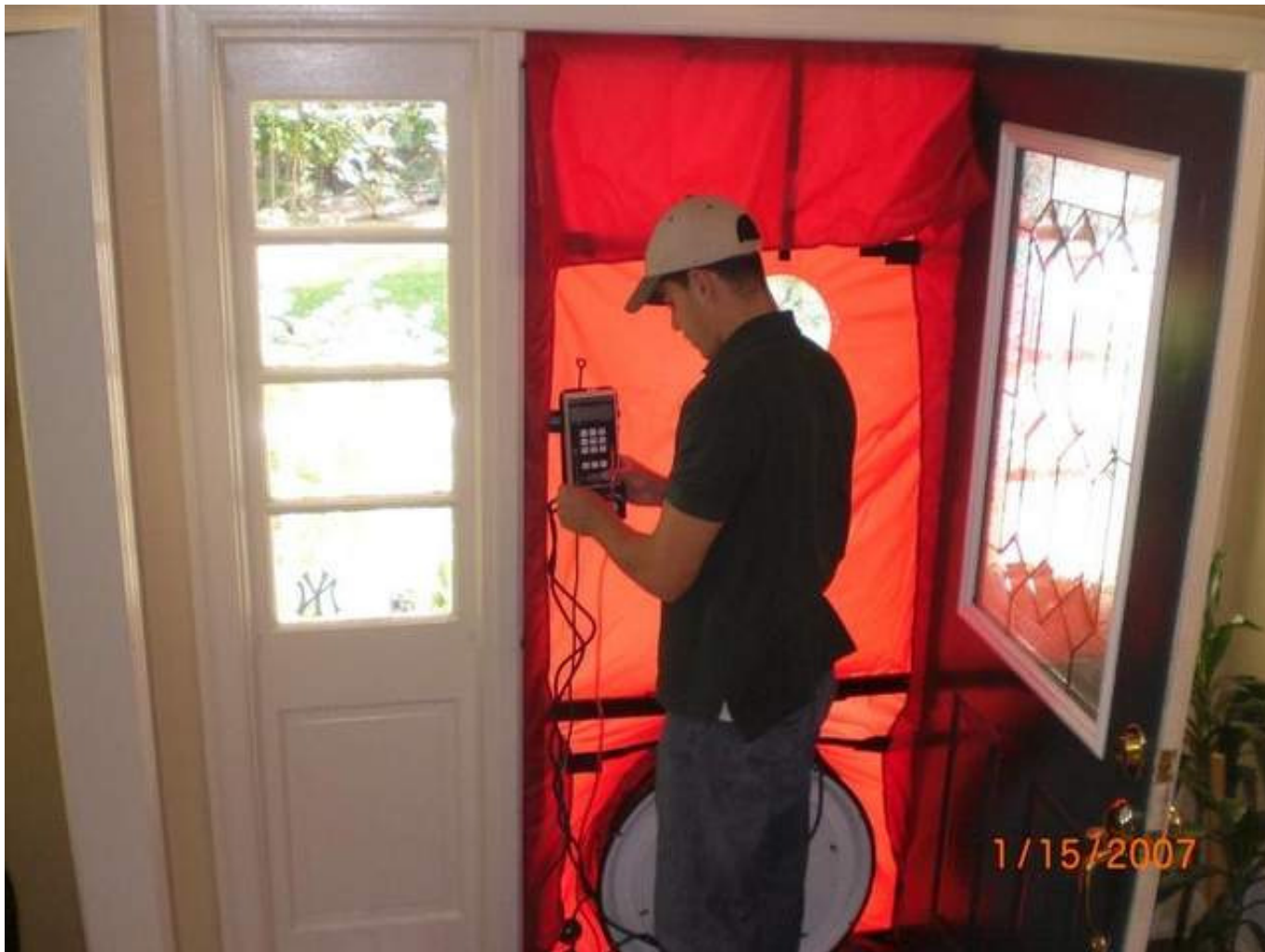
Jeremy Scott from Energy Management Solutions sets up CFM meter and fan to test amount of air leakage. / Photo courtesy of Jason Scher
